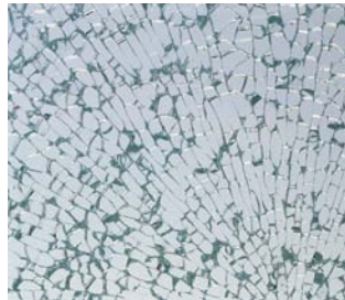
Fracture tempered glass
